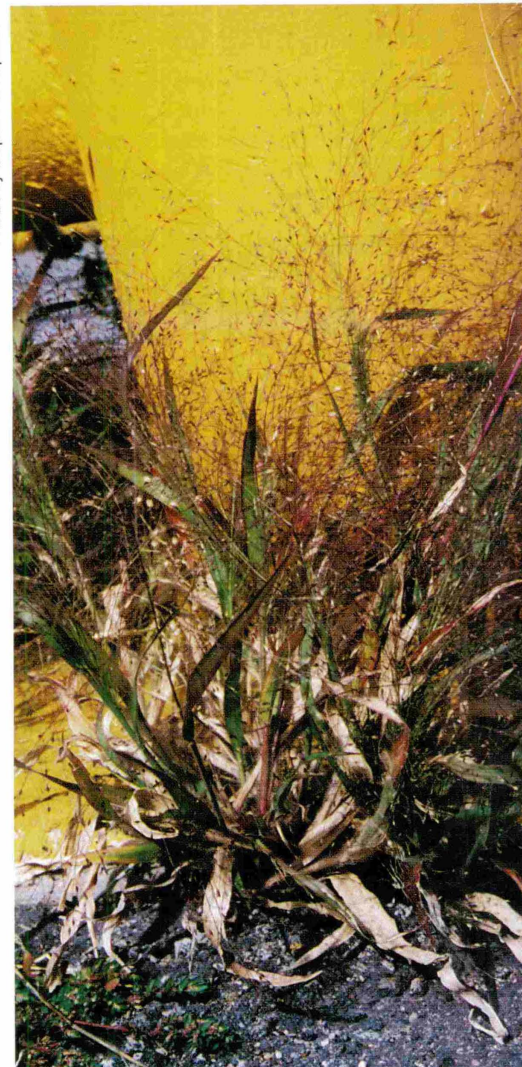
Witchgrass growing out of cracks in concrete.
