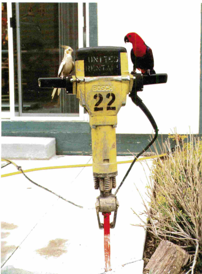
Taco and Tiki discuss the next step in the construction process. They are on a pavement breaker, which we used to break away some of the original patio slab to dig the 30 inch footer on the north side of the sunroom.
