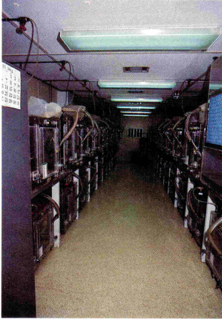
Banks of isolet cubicals are individually ventilated with filtered air and exhausted to the outside.
