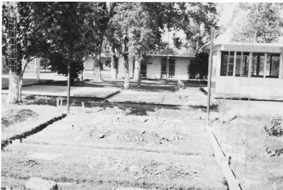
A foundation of concrete footing starts the UAT aviary structure on the UAT campus.
