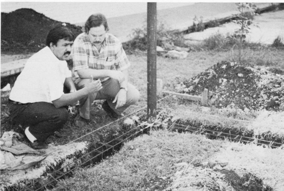
AFA's president Jack Clinton-Eitniewar (right) inspects the foundation of UAT's new parrot aviary in Ciudad Victoria, Mexico with Mario Vasquez, UAT's project coordinator. Construction of the aviary was due to financial support provided by several avicultural organizations.
